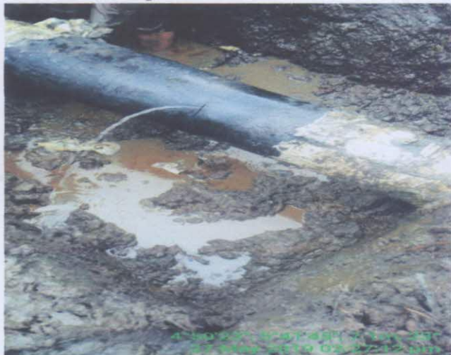
FIG C-D: Incident point on exposure
